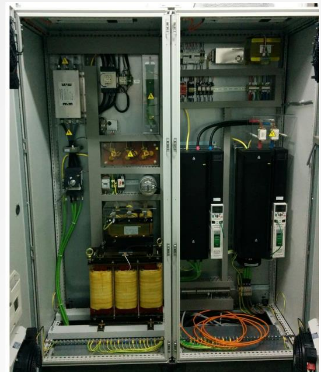
Mutriku control cabinet
